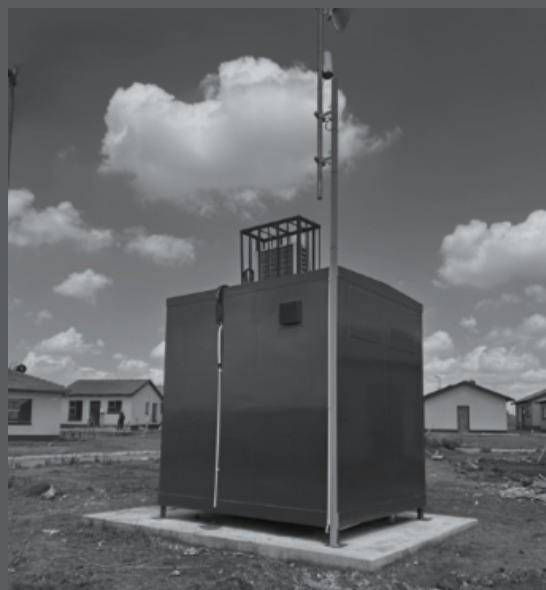
Figure 4. Vukela fibre network Point of Presence infrastructure located within communities, enabling a faster and more reliable broadband experience.
